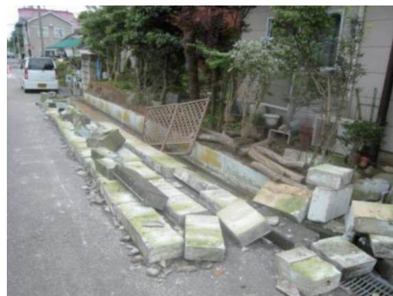
Collapsed stone wall
