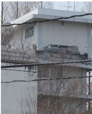
Top floor of 4-story building sustained damage
