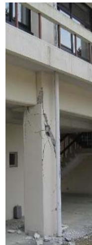
1st-floor support column in 2-story building fractured
