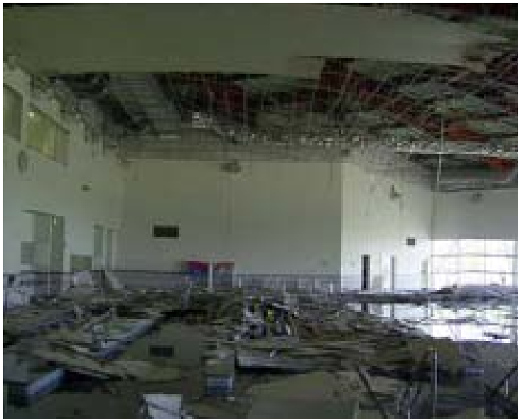
Collapsed ceilings at an indoor swimming pool (After the earthquake damage report of Ministry of Land, Infrastructure, Transport and Tourism)
