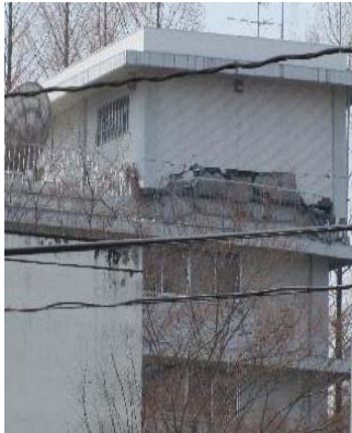
Top floor of 4-story building sustained damage
