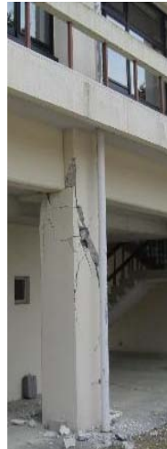
1st-floor support column in 2-story building fractured
